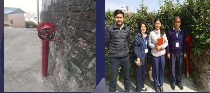
Dry Riser Laying Works for Fire fighting at different places of KMC
